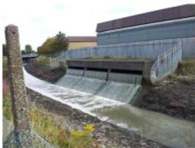
Unsatisfactory Intermittent Discharges (UIDs)
